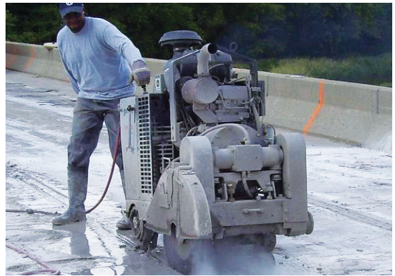
Examples of roadway cutting
